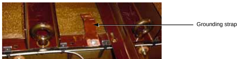
Figure 9: Core Ground Strap Location
