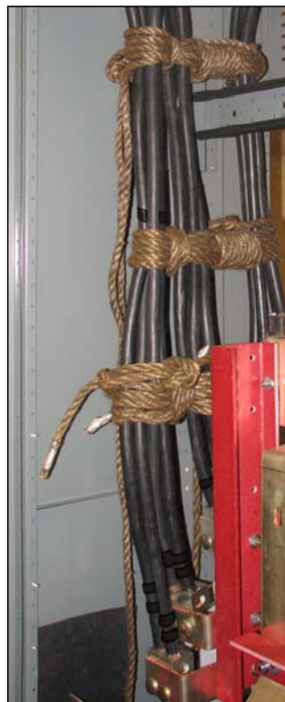
Figure 24 – Cable Restraint Example
