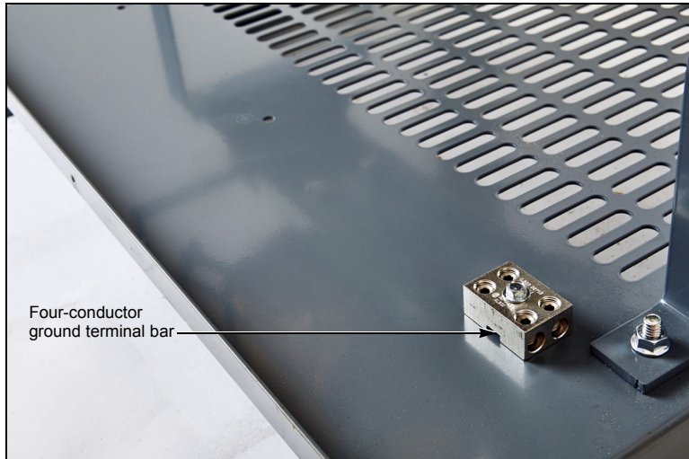
Figure 24: Four-conductor Ground Terminal Bar
